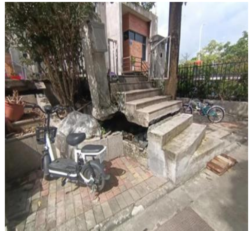
Figure 7: Examples of LS consequences. Top, the stairs broken in Nansha district
